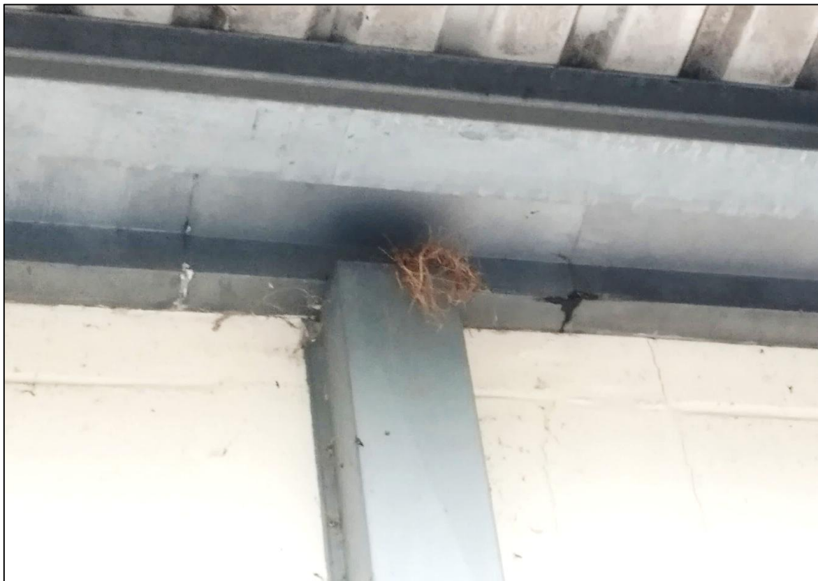
Abb. 4-1: Nistmaterial an Vordach
